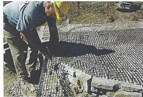
8. Cut the geo grid at the parting line near the face of the block for curved walls.
